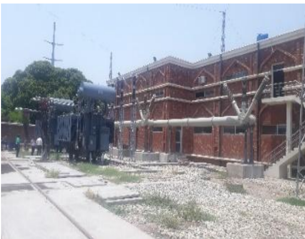
132kV GIS Sheranwala Grid
