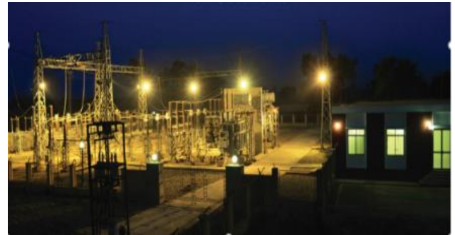
132kV AIS Machleod Ganj Grid
