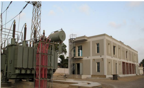
132kV GIS Mehmoodabad Grid cont.
